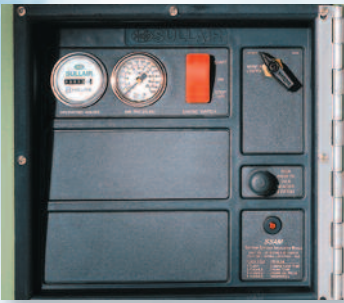
Curbside Instrument Panel Featuring SSAM Shutdown System & Annunciation Module.
