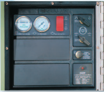
Curbside Instrument Panel Featuring SSAM Shutdown System & Annunciation Module.
